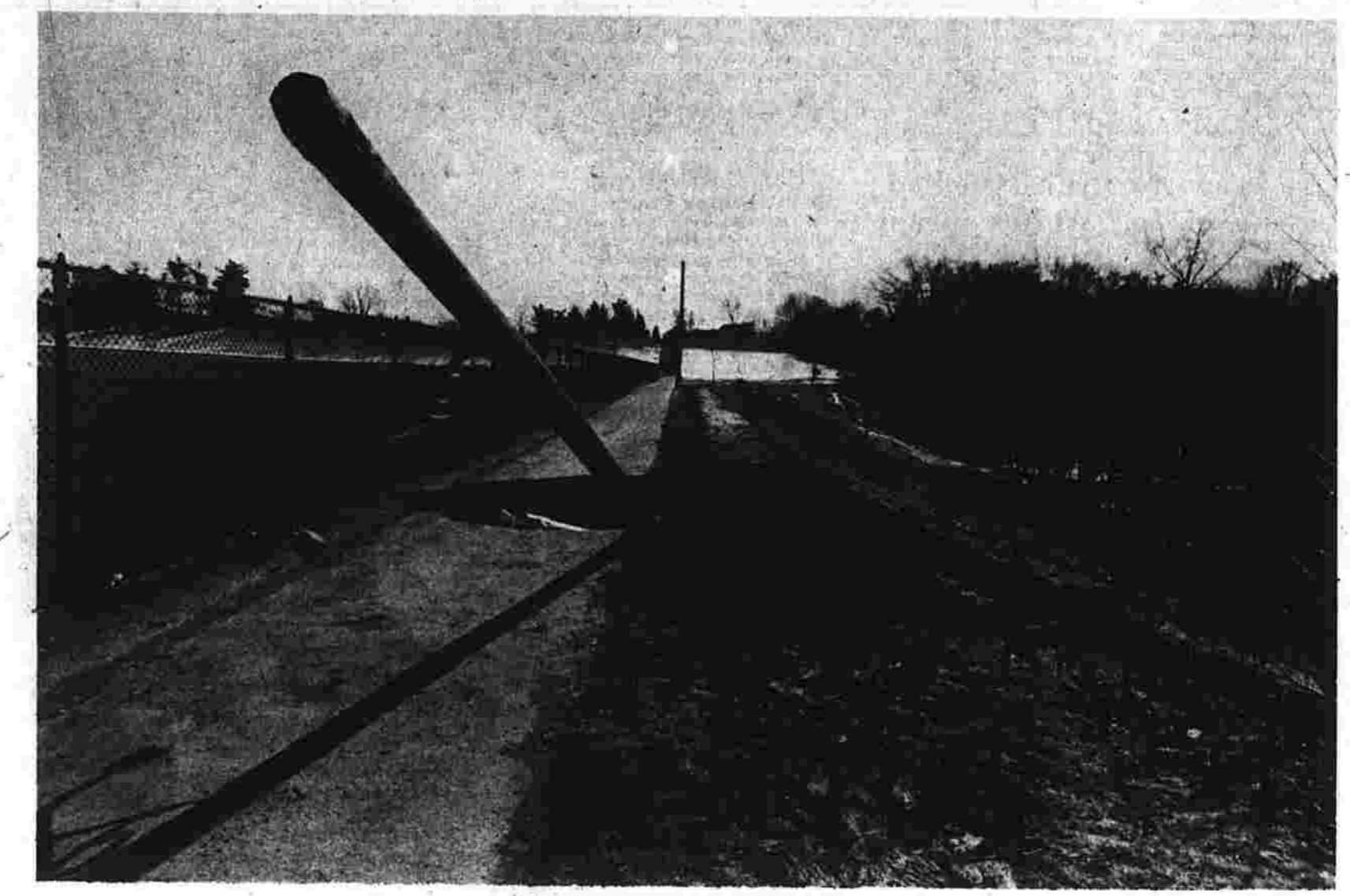
Hole Where the Walkway Was Recent heavy rains and a leak in an underground conduit next to Memorial Field at Manchester High School combined to wash out this substantial area outside fence on the west side of the field. The conduit is part of a system for removing surface water from the field and feeding it into Bigelow Brook. According to Charles Crocinni, assistant superintendent of buildings and grounds with the Board of Education, the pipe will be repaired and the area rebuilt by the town highway department. The pole, which lights the path leading to the tennis courts on Center St., will have to be reset, Crocinni says. The repairs will probably be completed by the end of the week, according to Crocinni. (Herald photo by Pinto)
